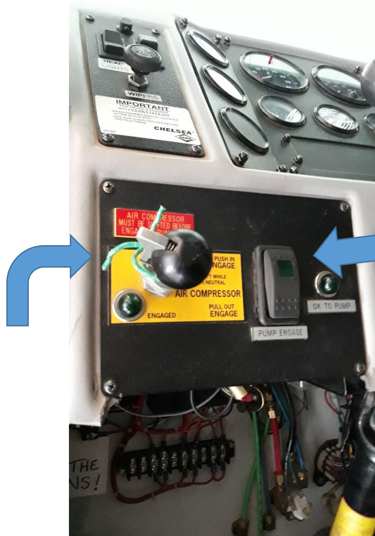
Compressor control switch
