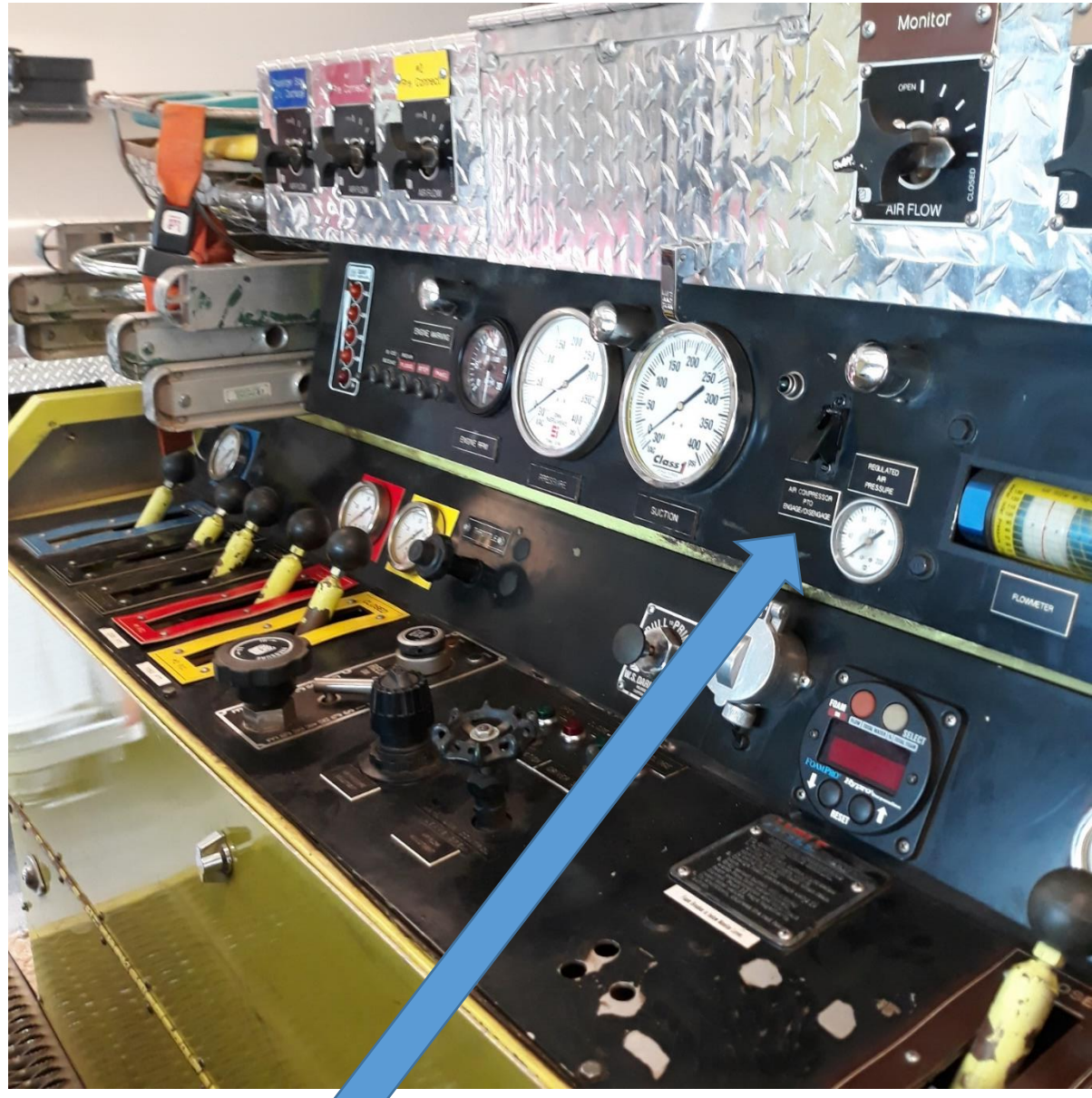
Air Compressor Controls
